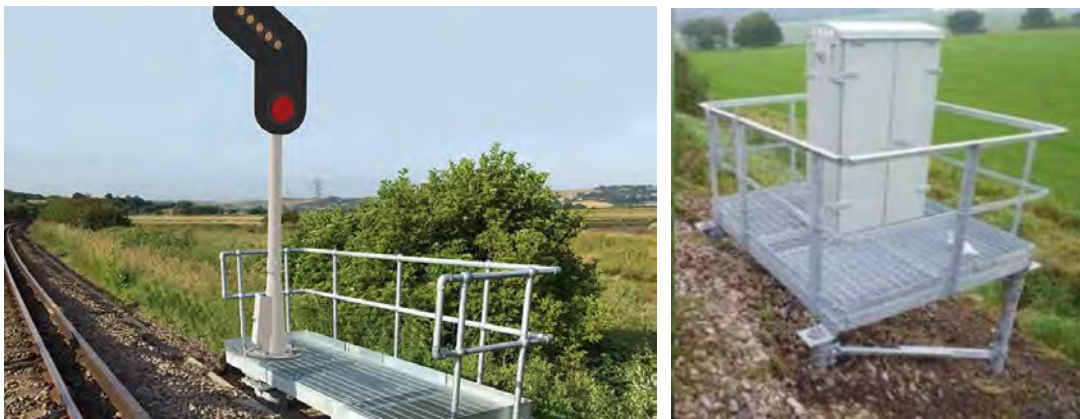
Figure 4-13 Signal and LOC installed on a platform
