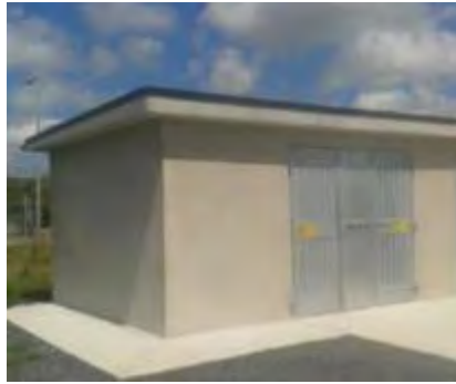
Figure 4-37 Example of an MV substation
