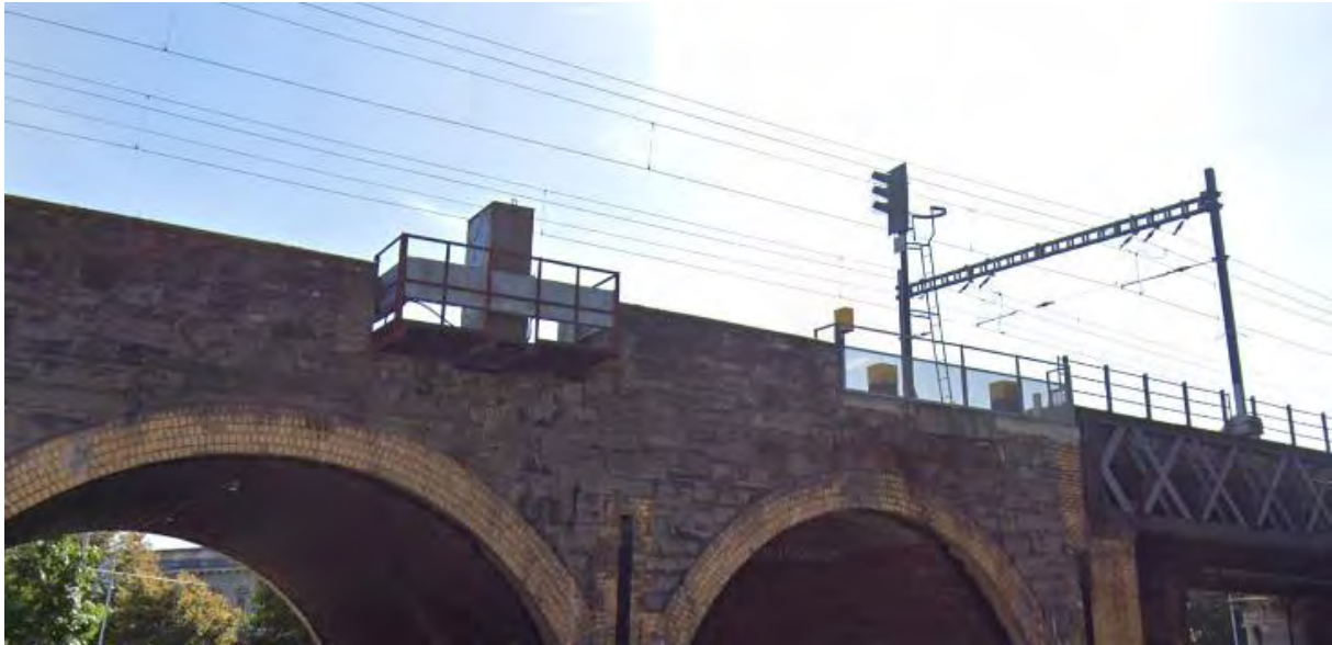
Figure 4-14 Signalling equipment installed on a bridge platform.
