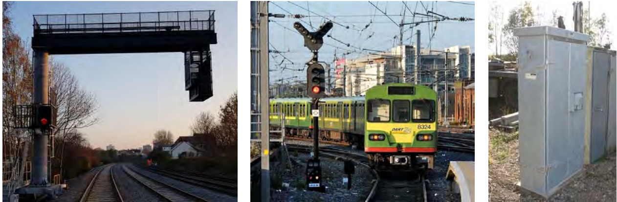
Figure 4-10 Sample DART+ West signalling infrastructure (cantilever, signal, LOC, from left to right)
