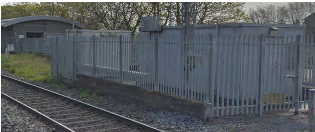
Figure 4-6 Example equipment cabinet
